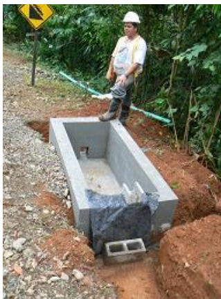
Water pressure regulator infrastructure
